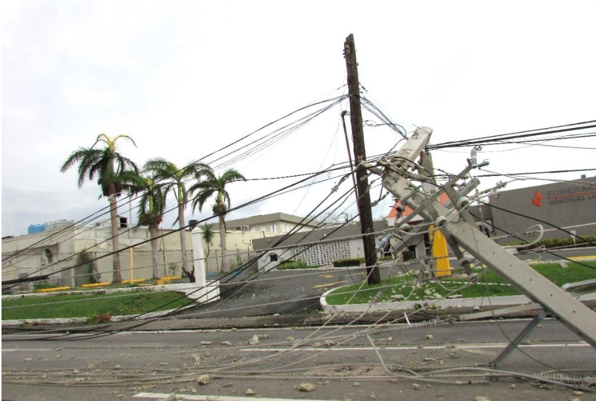
Figure 23 - Fallen wooden and concrete electric distribution pole at Puerto Rico Highway 65
